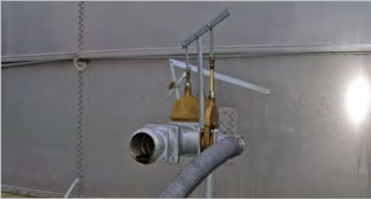
Entnahmestation Withdrawal station
