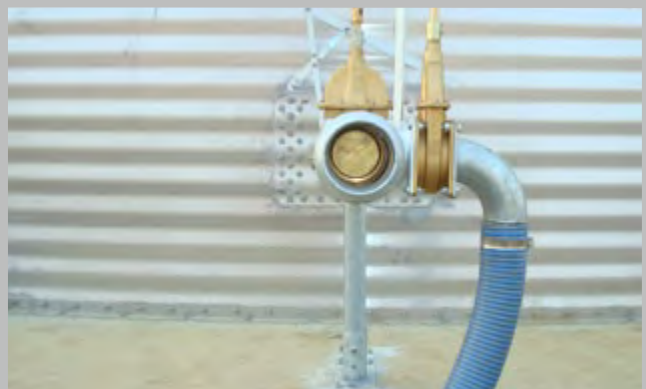
Entnahmestation Withdrawal station
